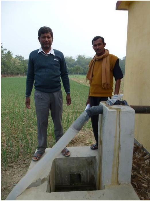
(a) Outlet from the tubewell with the flow meter located in the pipe at the top of the concrete pillar, Shikara-I LDTW irrigation scheme, West Bengal
